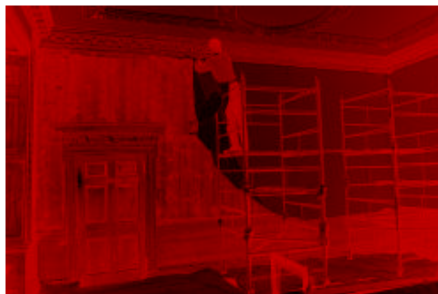
2. Hanging the polyester textile. Showing the wall surface constructed of wooden planking.
