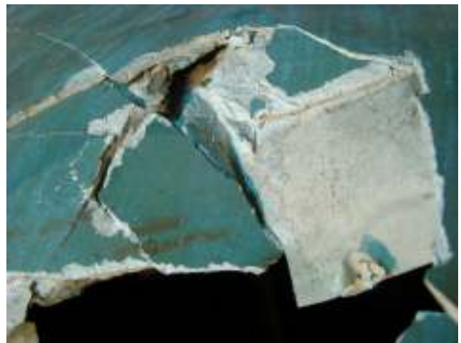
Fig. 2. Detail showing breakage and structural loss
