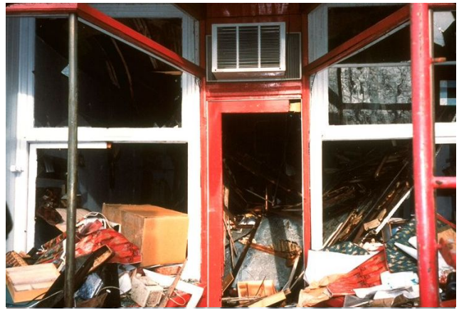
Fig. 2. The store front after the fire
